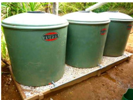
Some of the installed water tanks at Yarik.
