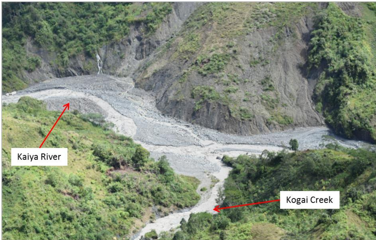
Figure 4-20 Kaiya River bank failure opposite the Kogai Creek Confluence
