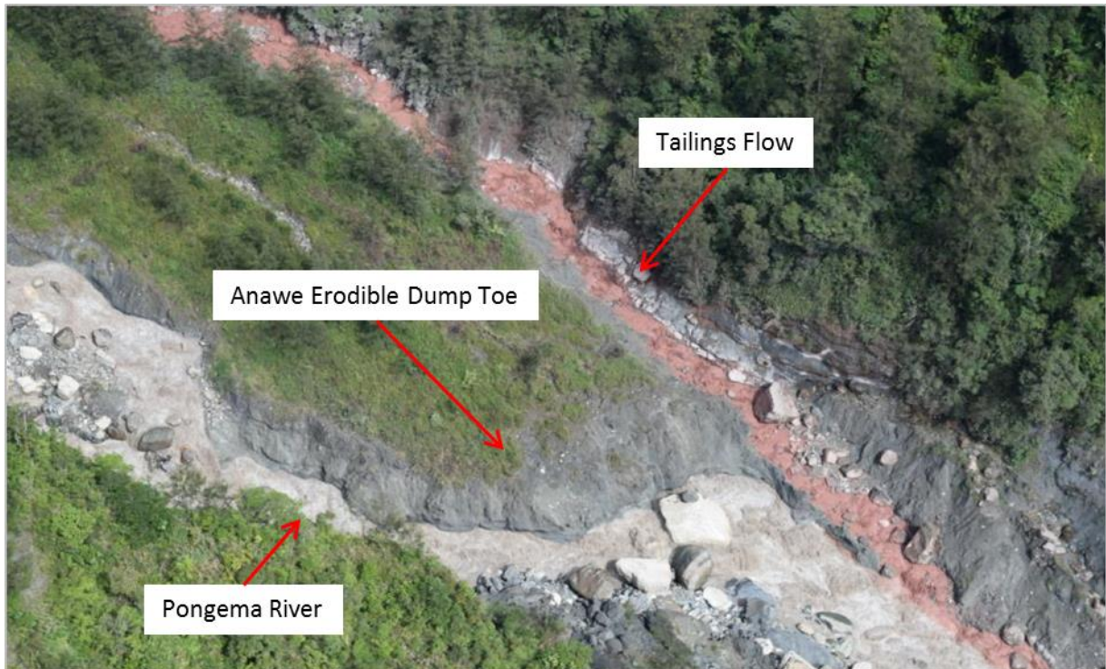
Figure 4-18 Anawe erodible dump toe
